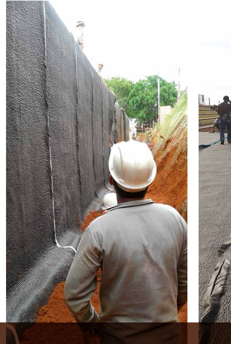
Railway track drainage
